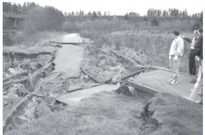
Earthquake damage to the trail at the Interpretive Center. Courtesy of Thurston Regional Planning Council, 2001.
