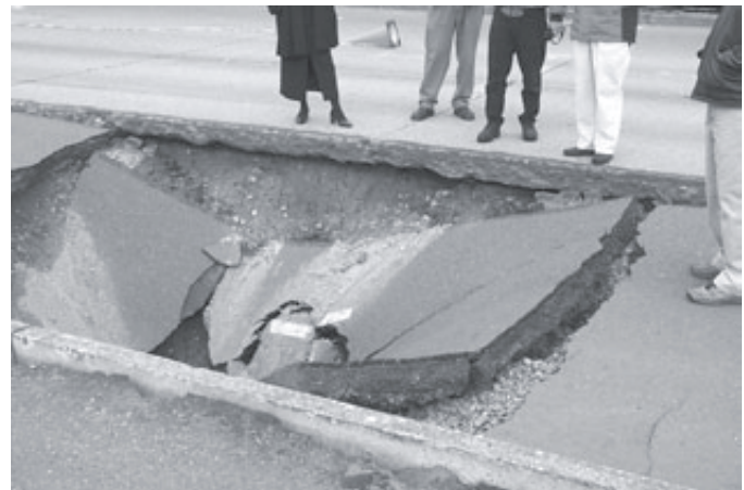
Sinkhole caused by damaged culvert on Deschutes Parkway. Courtesy of Thurston Regional Planning Council, 2001.
