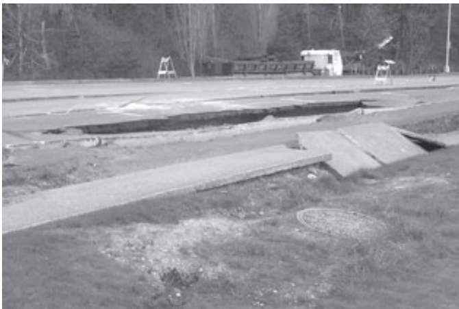
Damaged road bed and sidewalk on Deschutes Parkway. Courtesy of Thurston Regional Planning Council, 2001.
