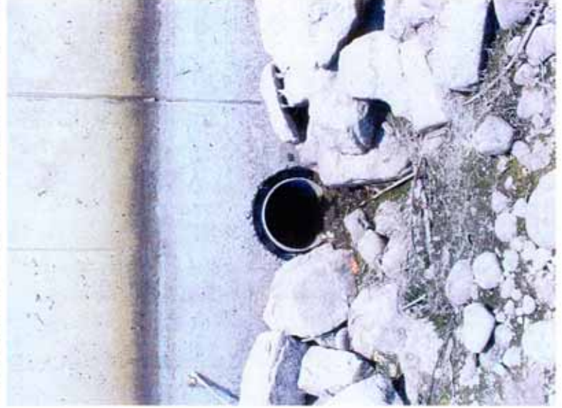
Above: Seepage with a sheen along Heritage Park
