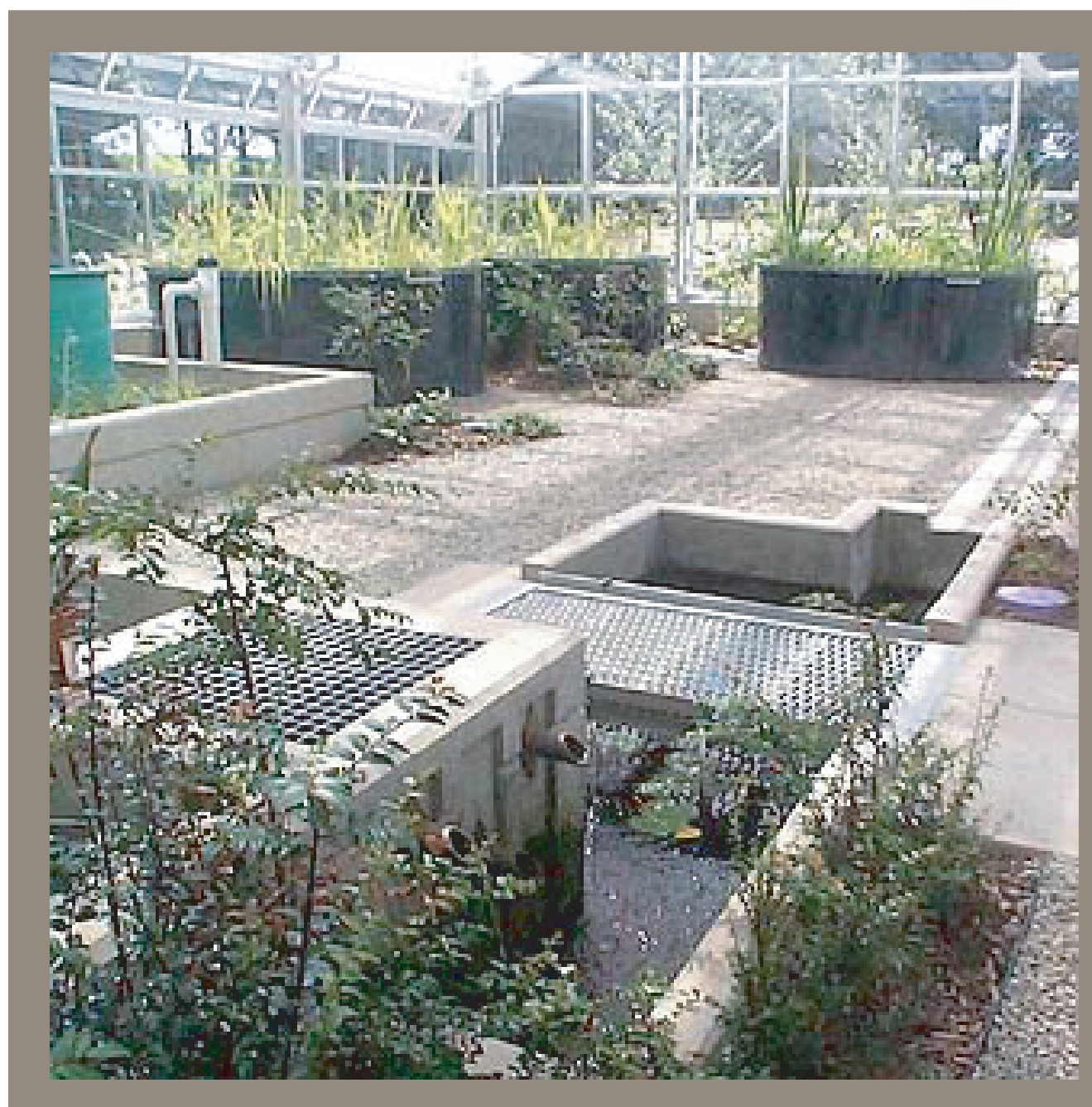
Living Machine At Islandwood, WA
