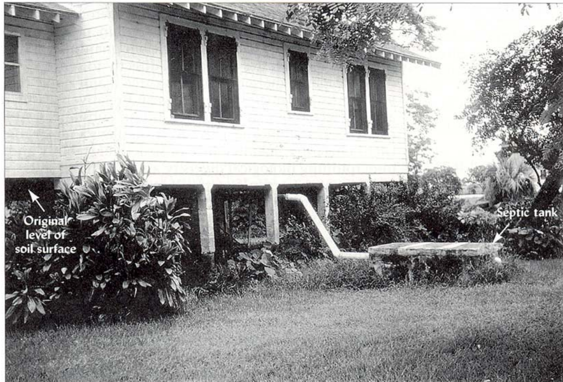
FIGURE 12.32 Soil subsidence due to rapid organic matter decomposition after artificial drainage of Histosols in the Florida Everglades. The house was built at ground level, with the septic tank buried about 1 m below the soil surface. Over a period of about 60 years, more than 1.2 m of the organic soil has “disappeared.” The loss has been especially rapid because of Florida’s warm climate, but artificial drainage that lowers the water table and continually dries out the upper horizons is an unsustainable practice on any Histosol. (Photo courtesy of George H. Snyder, Everglades Research and Education Center, Belle Glade, Fla.)
